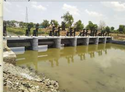
Tiwasa project: Automatic Gates in open position
