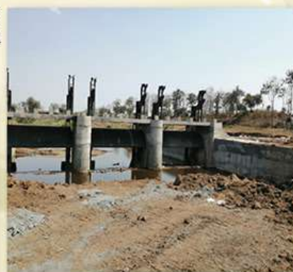
Jamni project: Automatic Gates in open position
