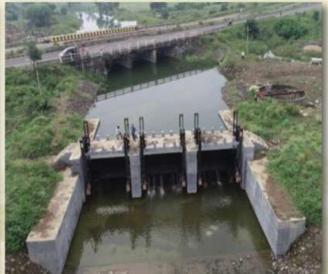
Sarwadi project: Automatic Gates (Radial)
