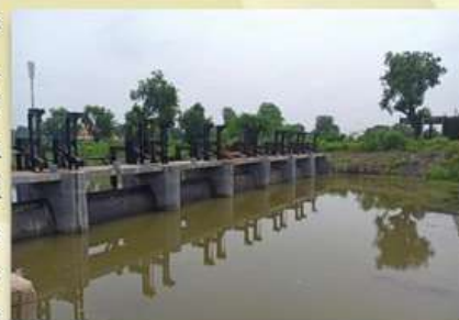
Tiwasa project: Automatic Gates (Radial)
